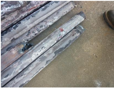
Boiler Tubes (before)
