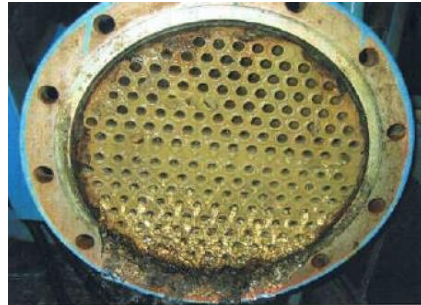
Compressor after cooler with scale
