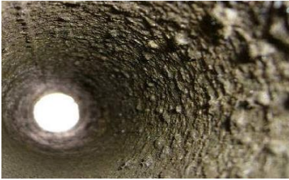
Feed Line to compressors with scale deposition
